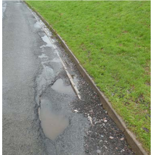
People's Park pot holes: a watery trap for unsuspecting motorists
