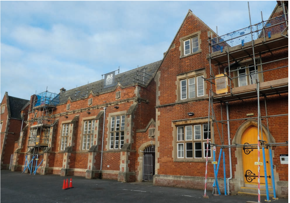
College House at Western Road opened in 1859 as a boys' grammar school. Urgent works are soon to start to repair roof and other structural defects.
